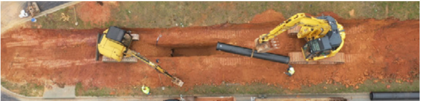
Augusta Road Water Main
