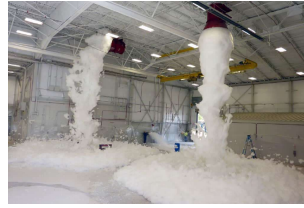
Foam Extinguishing Systems
