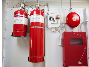
Dry Chemical Extinguishing Systems
