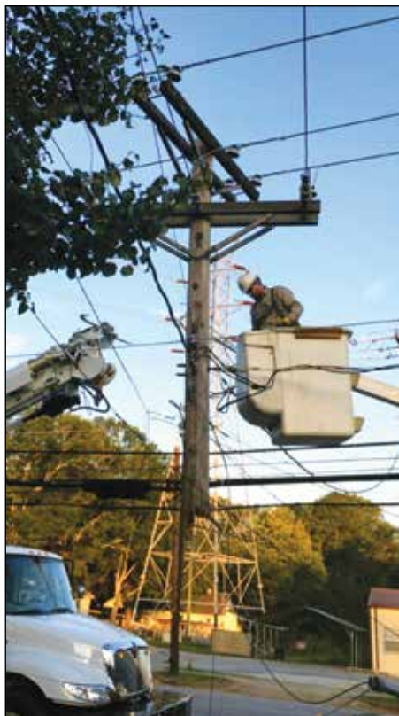
Kalen Sipes describes line work as a rewarding job that allows him to help others in difficult situations. Photo: Laurens Commission of Public Works.
