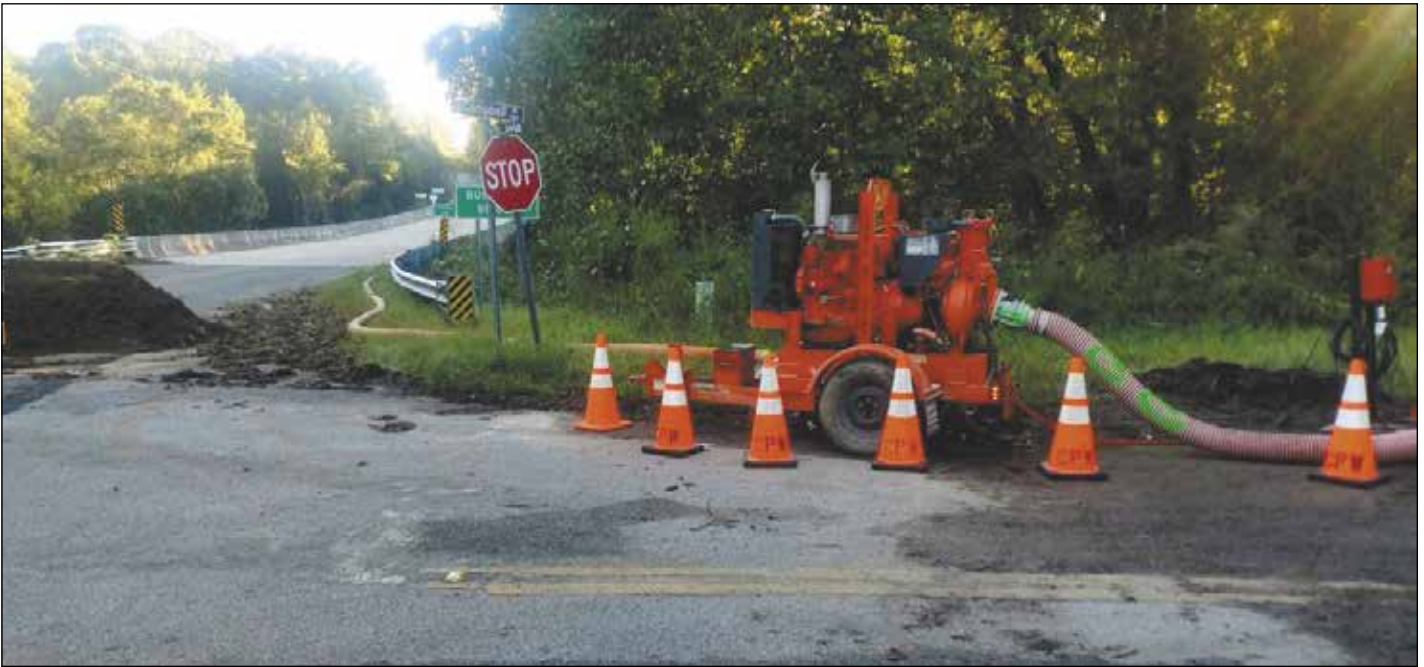
The City of Camden came to the aid of the Town of Chesterfield with a bypass pump when flooding washed out a 12-inch sewer line.
