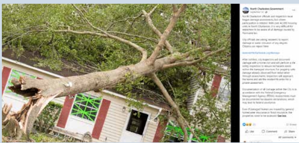
After Hurricane Ian, North Charleston used social media to spread the word on how city inspectors were handling damage inspections, and how residents could report damage. Photo: City of North Charleston.
