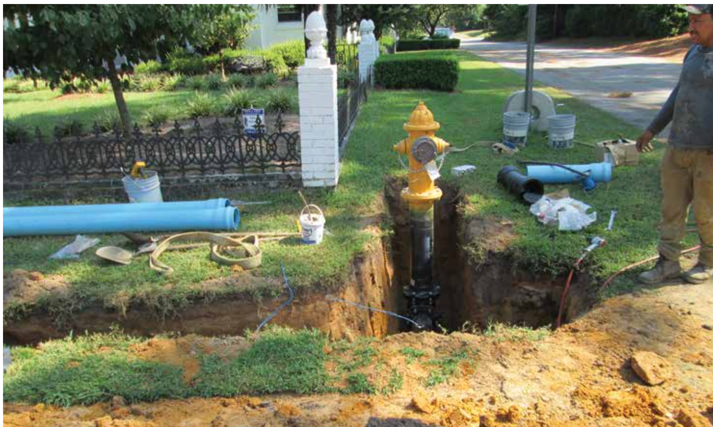
While replacing most of its water infrastructure, the City of Cayce mobilized its contractors, staff and elected officials for an equally massive communications effort. Photo: City of Cayce.
