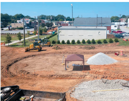
Improvements to McKinney Park, now connected to Main Street, form part of Woodruff's investments in its downtown. Photos: City of Woodruff.
