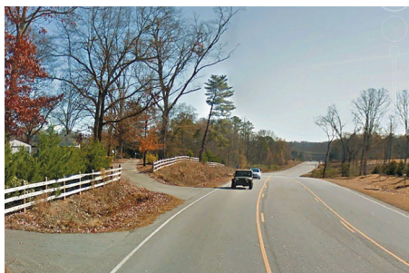
Improvements to Stenhouse Road in Simpsonville are seen during and after construction. Photos: City of Simpsonville.
