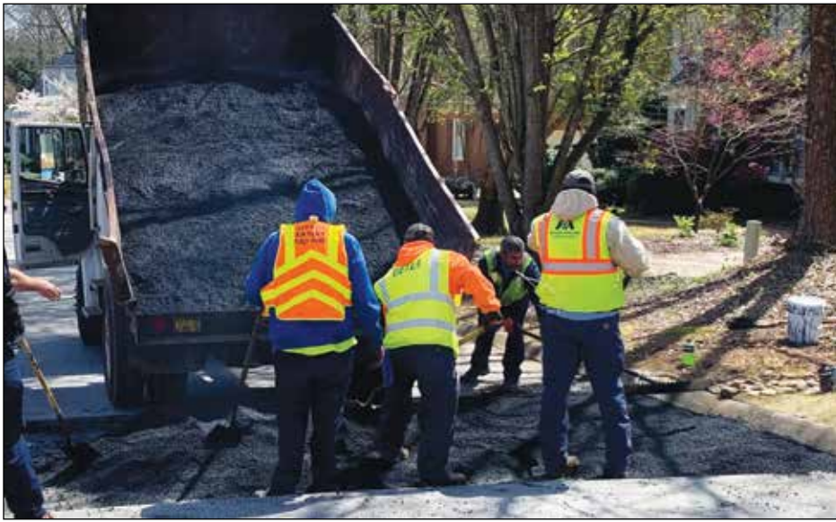
Easley's Public Works Department has added road paving to its list of responsibilities. Photo: City of Easley.
