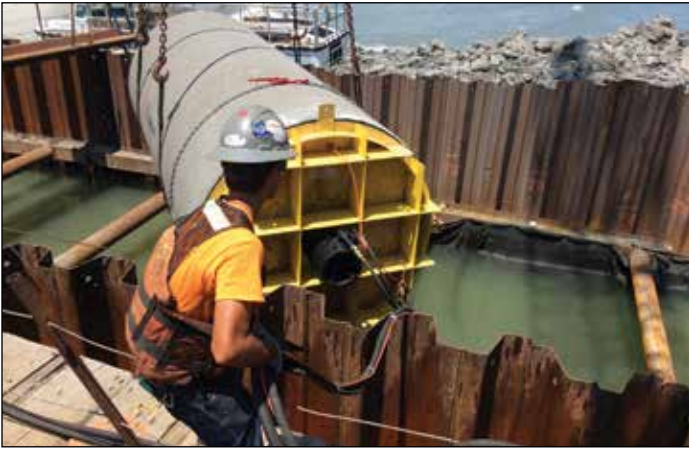
Myrtle Beach built the 4th Avenue North Ocean Outfall project to maintain high water quality while reducing beach erosion. Photo: City of Myrtle Beach.
