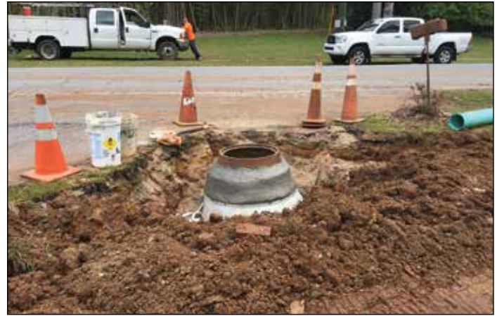
The Town of Lockhart used a grant to address a sanitary sewer overflow from a blockage in an old, deteriorated line. Photo: Town of Lockhart.
