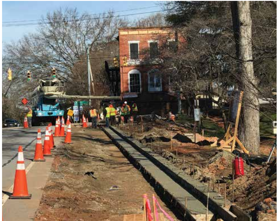
Crews install streetscape enhancements along North Mechanic Street in Pendleton. Photo: Town of Pendleton.
