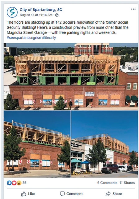
The City of Spartanburg shares photos and information about current development projects.
